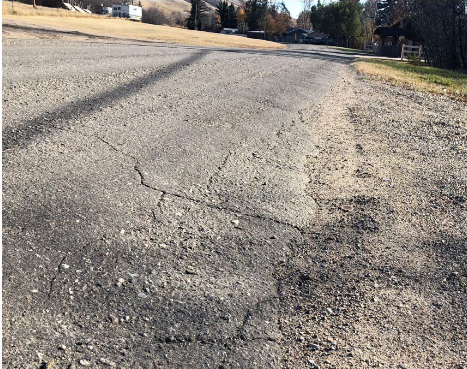
Figure 5: Pavement Conditions on Daniel Drive
